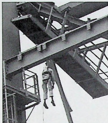
A German worker dies when scaffolding collapses
