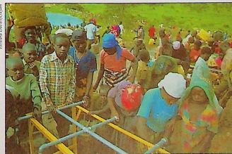
Oxfam water installation at Bwako camp, Tanzania.
