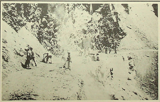
Above The road between Tehri and Gansyali. The shoulders of the road are so loose that road gangs have continuously to clear away debris from the almost permanent landslips while buses wait their turn on either side of the bend.
