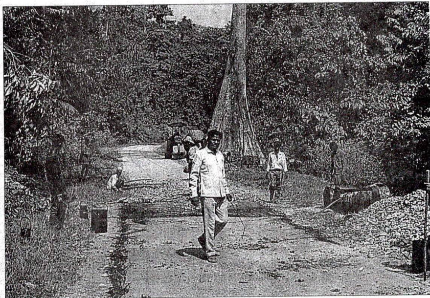
Maintenance work on the Andaman Trunk Road inside the Jarawa reserve. Large quantities of timber are burnt for the maintenance of the road.
